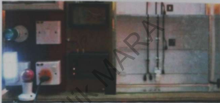
Figure 4.4: Flood Detection System in Third Stage Condition
